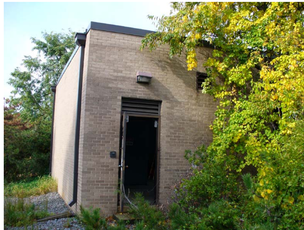
TIE BREAKER ACCESS
