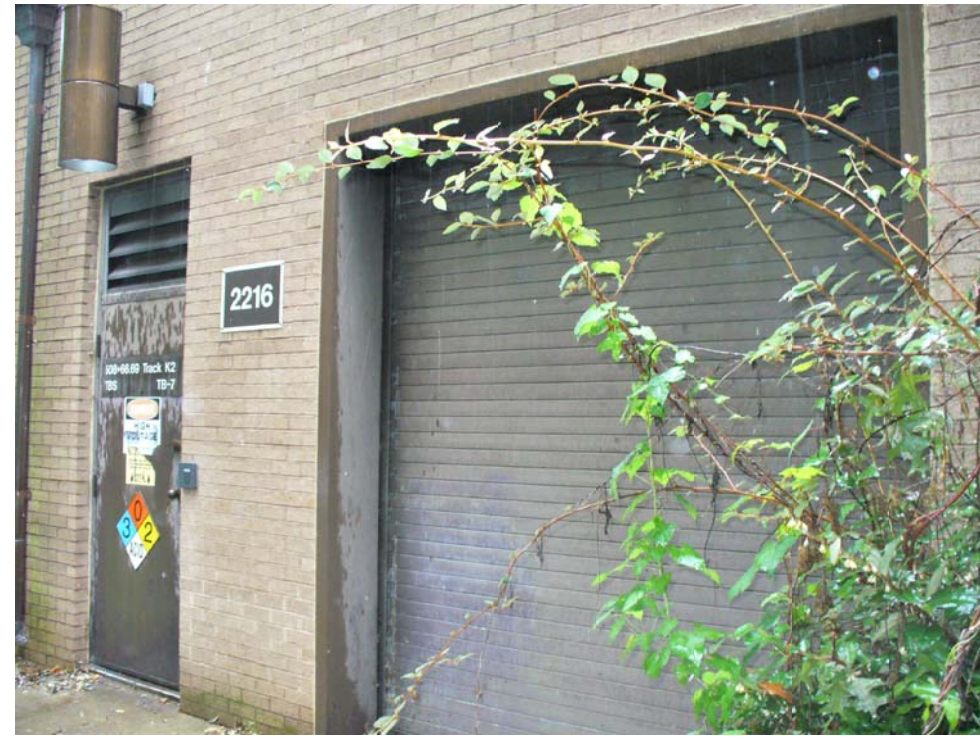
TIE BREAKER ACCESS
