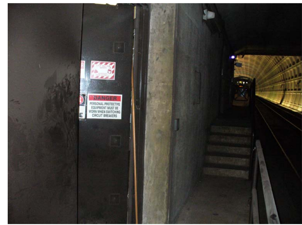
TIE BREAKER ACCESS
